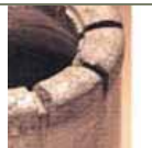
Loss of inside diameter
