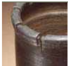
Cracks in the water ways
